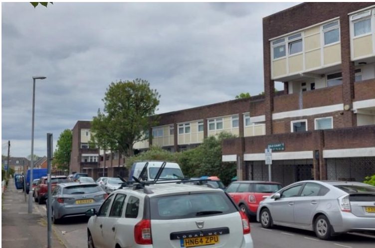
Dale Court in York Road: Note how brick parapets without weather capping have badly stained from descending dampness. The lightweight cladding is peculiar to this building
