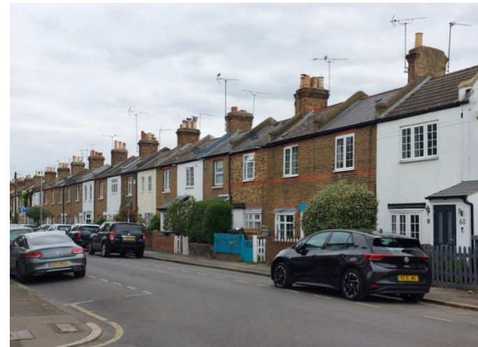
Victorian Cottages York Road: Terraced cottages in York Road that face the building York House in the previous picture to the left. Some are spoiled by plumbing on front elevation and others by chimney repair alterations and concrete roof tiles.
