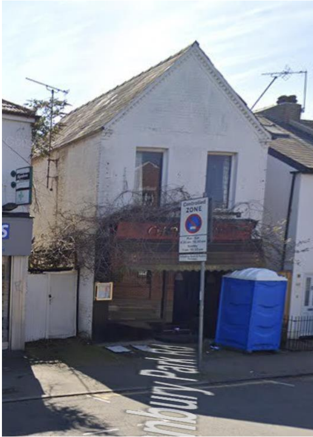
Dilapidated shop front 2019 with thanks to Google Streetview
